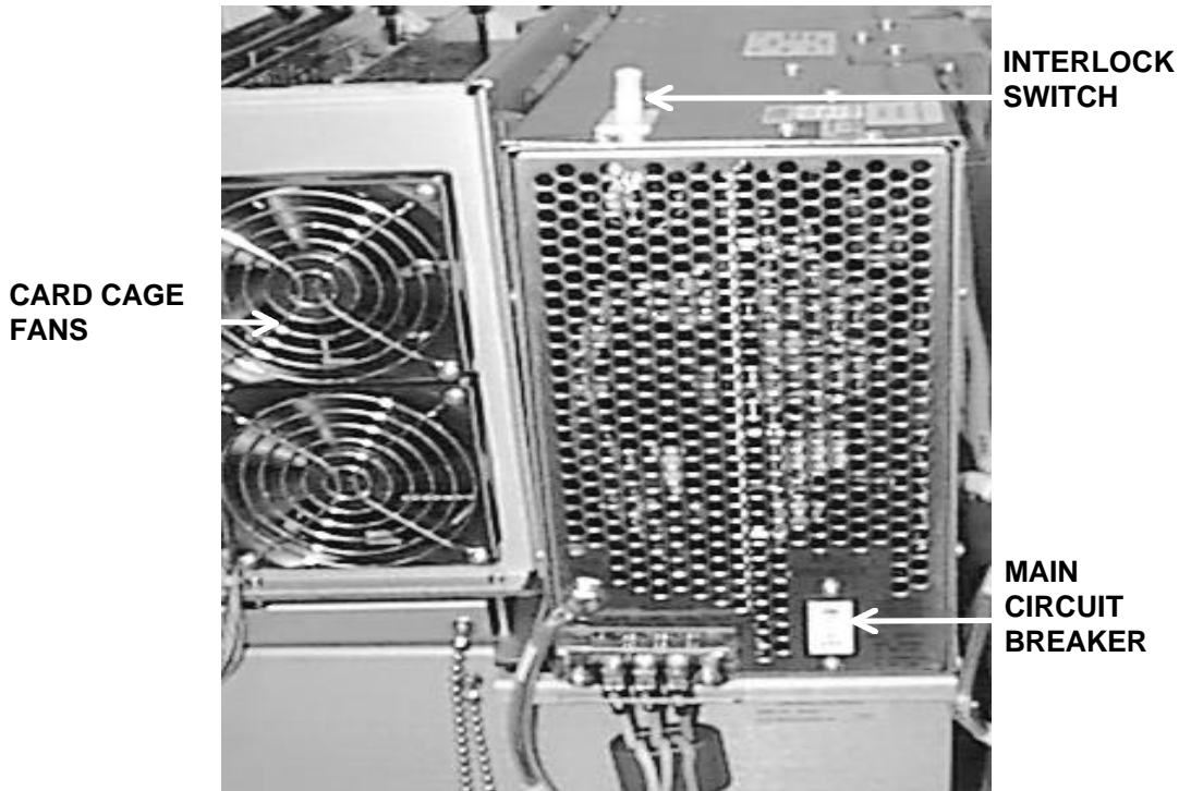
Figure 3-9. The main circuit breaker and interlock switch are on the right side of the system power supply.
